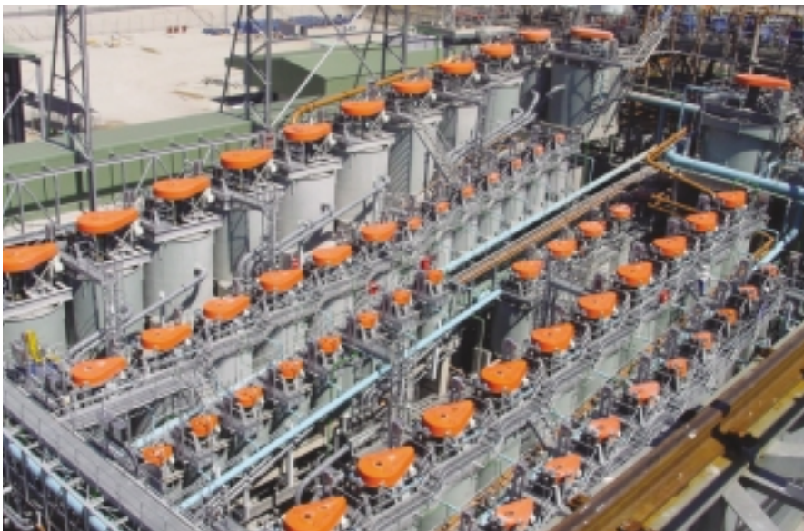
Flotation cells at the processing plant that serves Aquarius Platinum's Marikana mine. The plant was commissioned in November 2002.
