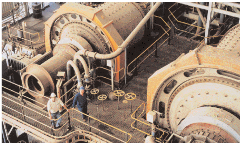
The mill at Barplats' recently reopened Crocodile River mine
